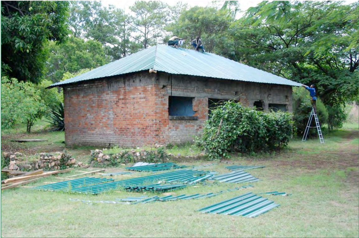
Roofing sheets go up on “The Cottage”. Guests may be able to stay in this house in the future
